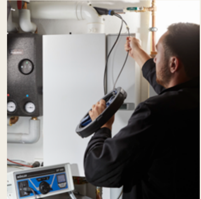
Leakage test of the flue gas system: In preparation for the test, the flue gas pipe is sealed at the top and bottom with sealing bubbles. This is very simple, as the bladders can be easily pushed through the pipe from below using a reel and then position them.
