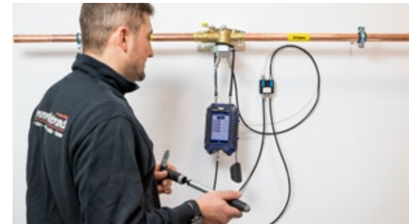
With the appropriate connection accessories, the newly installed gas pipe is simply pressurised with the test pressure for the stress test (1,000 hPa).
