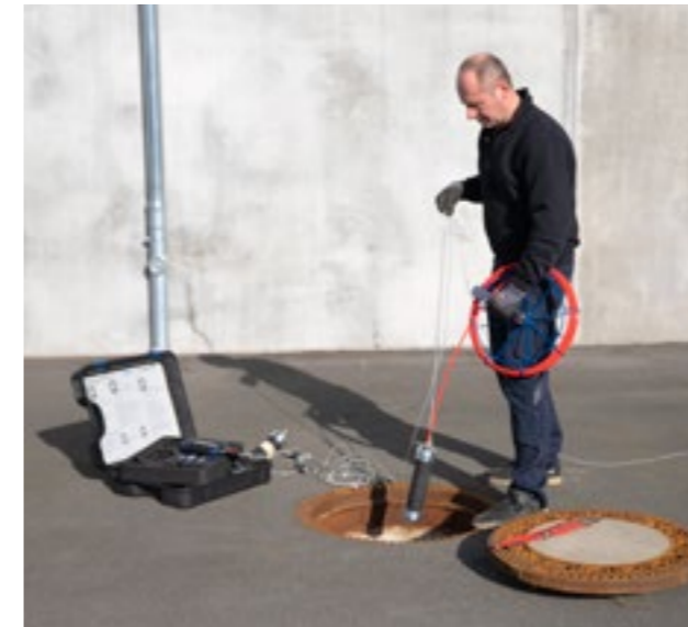
Prior to conducting the leak tightness test on wastewater pipes in accordance with DIN EN 1610, the test sections are sealed using bladders.
