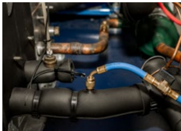
Connection hoses with ball valves for quick closing and opening of refrigerant flow.
